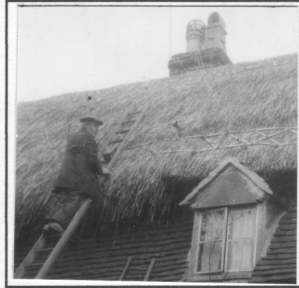
16. Thatching the roof of the cottage next to Brickwall Farm, early 1930s.
